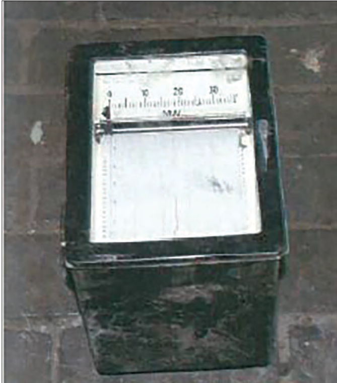
Figure 13.8 Recorder, range 0-36 MW, Manufactured by SIEMENS, 1956
