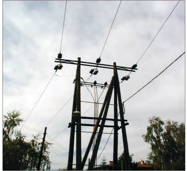
Figure 2.7 Transmission line 35 kV Banja Luka 1 – Petričevac
