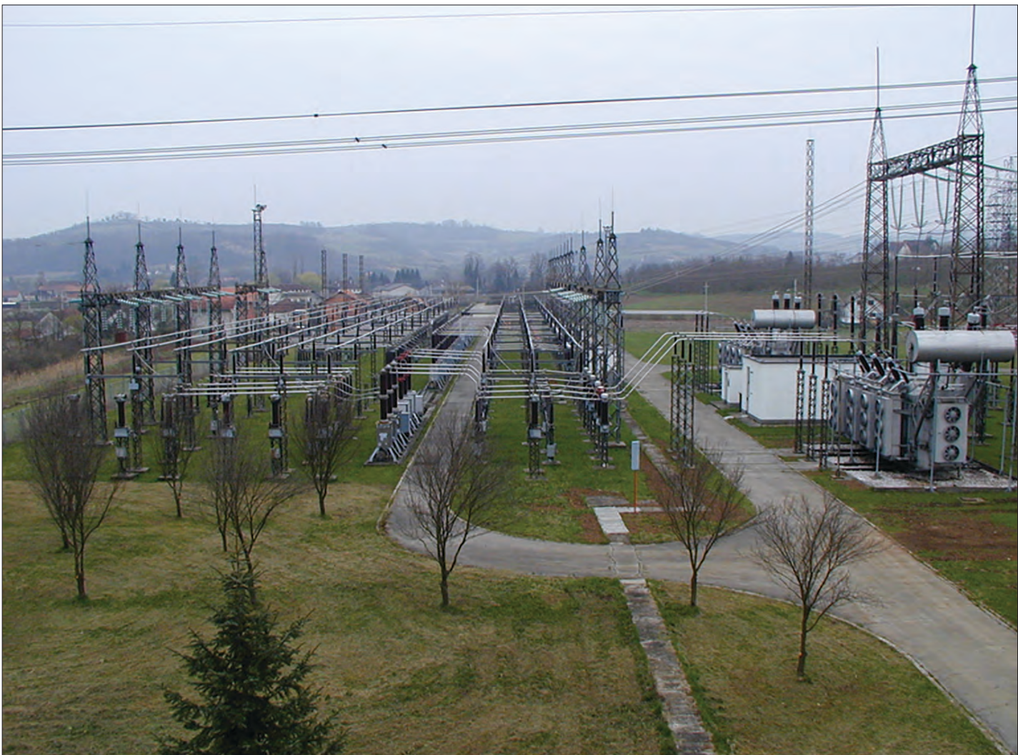
Figure 2.26 TS 400/110 kV Banja Luka 6
