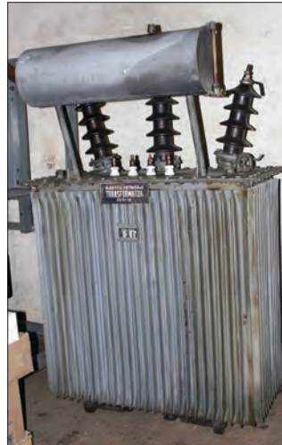
Figure 13.13 Transformer 35/04 kV (produced in 1956 by RADE KONČAR)
