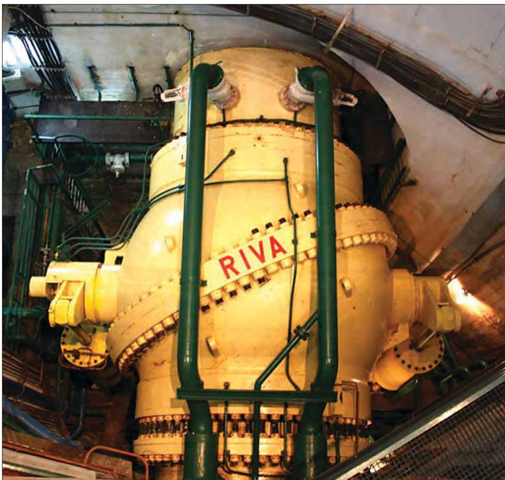
Figure 2.25 PS HPP Čapljina, turbine plant, in operation since 1979/80
