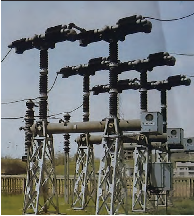
Figure 3.14 Energoinvest's high-power laboratory, a) protection breaker, 1985
