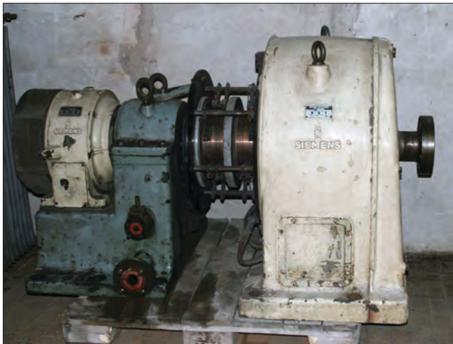
Figure 13.12 Generator exciter 32 MW (production 1956 SIEMENS)
