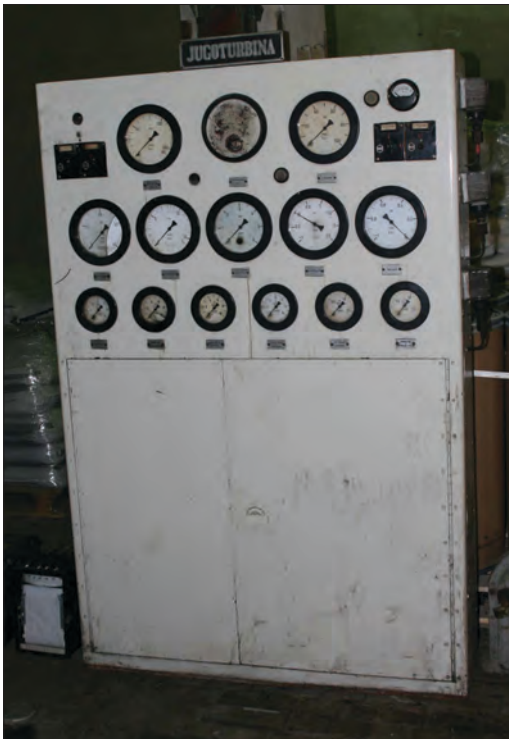
Figure 13.10 Instrument panel in front of the turbine for monitoring the operation of the 32 MW turbine (production 1956)
