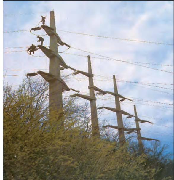
Figure 2.15 110 kV transmission line with concrete pillars
