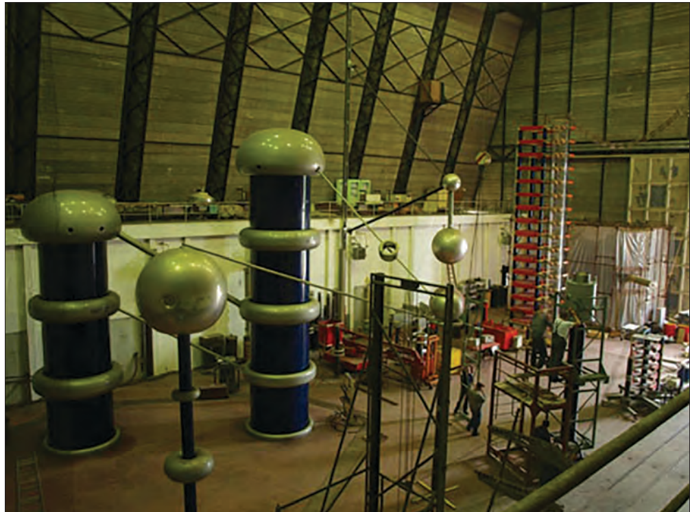
Figure 3.11 High voltage laboratory in Lukavica
