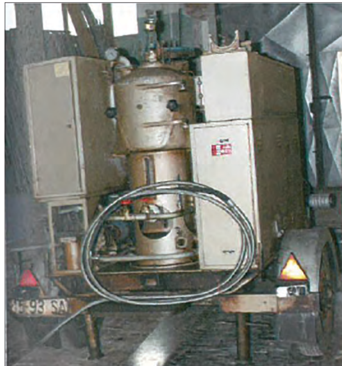
Figure 13.11 Transformer oil filtering machine, GALILEO MODEL 26 A512, in use since the 1960s
