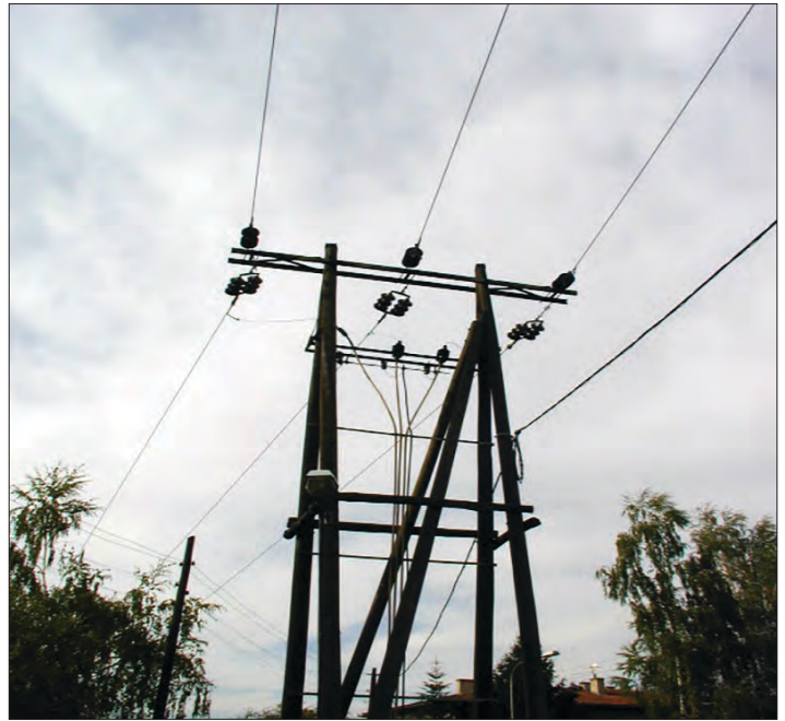
Slika 2.7 Dalekovod 35 kV Banja Luka 1 – Petrićevac
